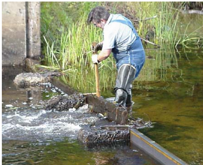
DNR maintenance specialist replacing wooden stop logs with steel channels at the Island Lake outlet dam in Crow Wing County (photograph by Ron and Judy Rolfe).
